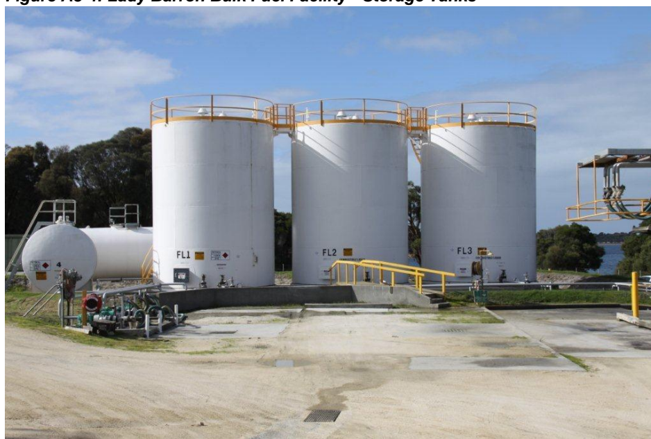
Figure A3-4: Lady Barron Bulk Fuel Facility - Storage Tanks
