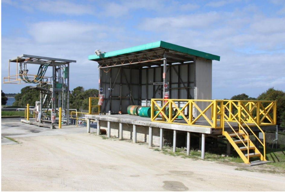
Figure A3-5: Lady Barron Bulk Fuel Facility – Pump Station
